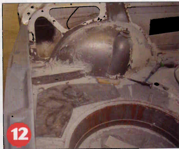
12) The hatch and spare wheel area was then prepped for its new interior panels and final finishing work
